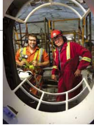
ASI Marine's hyperbaric tunnelling specialist, Jerry East, and technician Thomas Koop standing on a TBM's air lock platform.
