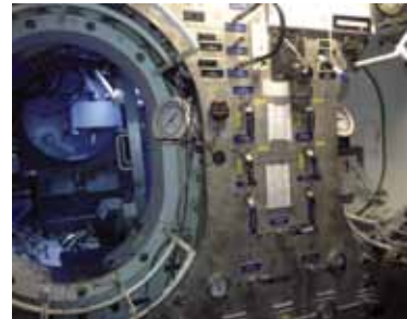
A TBM air lock.
